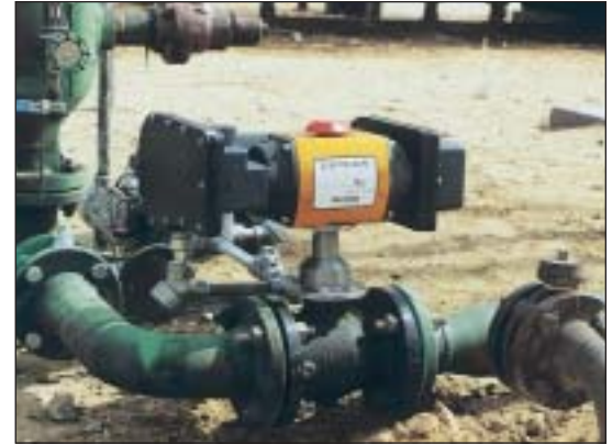
Oil production water dump application
